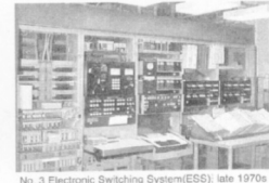
No. 3 Electronic Switching System (ESS), late 1970s
