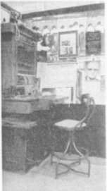
"Timbuktu Telephone Company" and magreto switchboard, part of the Ted Hewitt Collection
